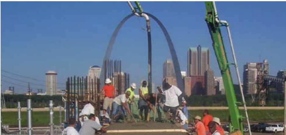
Construction of the Mississippi River Overlook at Malcom W. Martin Memorial Park, East St. Louis, IL.
