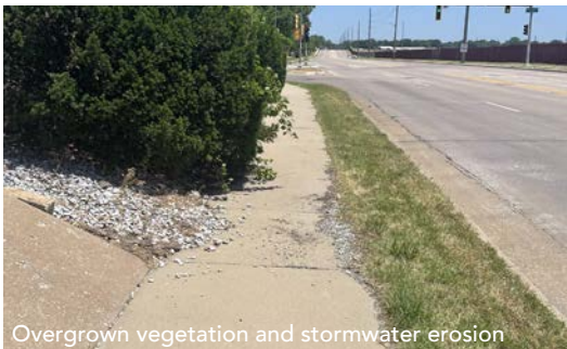
Overgrown vegetation and stormwater erosion
