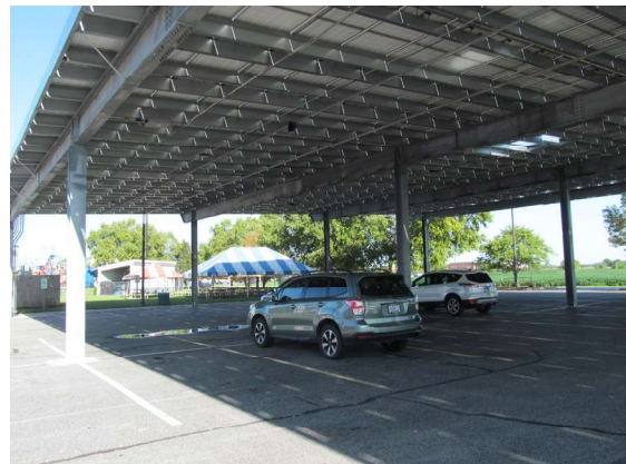
Solar Panel Shade Structure Missing Panel
