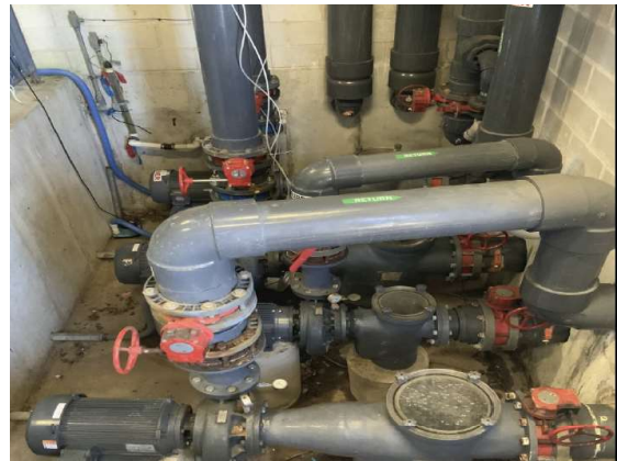
Some Repairs Needed on Aqua Park Systems
