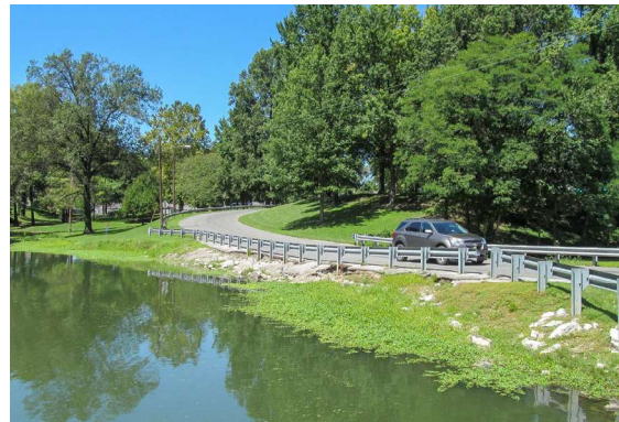
Erosion Where Lake Crosses Road
