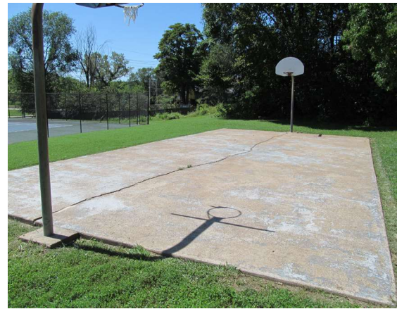
Glidden Park Basketball Court Needs Repair
