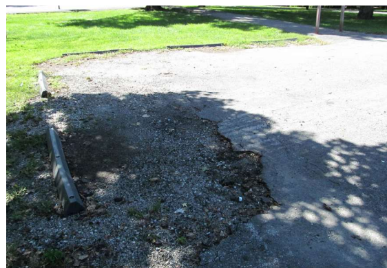
Parking lots need repaving and striping
